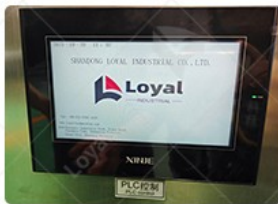
1. PLC control system
