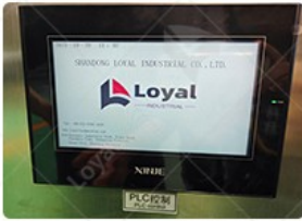
1. PLC control system
